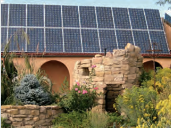
Grid-tied solar array at Cliffrose Garden Center - Cortez, CO
